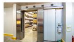
Refrigeration and cooling
