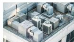
Heating, ventilation and air conditioning (HVAC)
